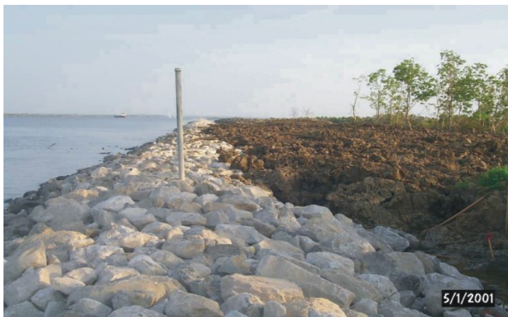
This completed rock riprap structure was placed adjacent to the existing shoreline to buffer it from the erosive forces of wake-induced wave energy.
