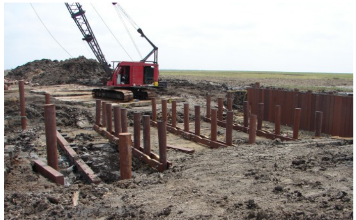
Early stages of the construction of a water control structure to move freshwater to brackish marshes to the south.
