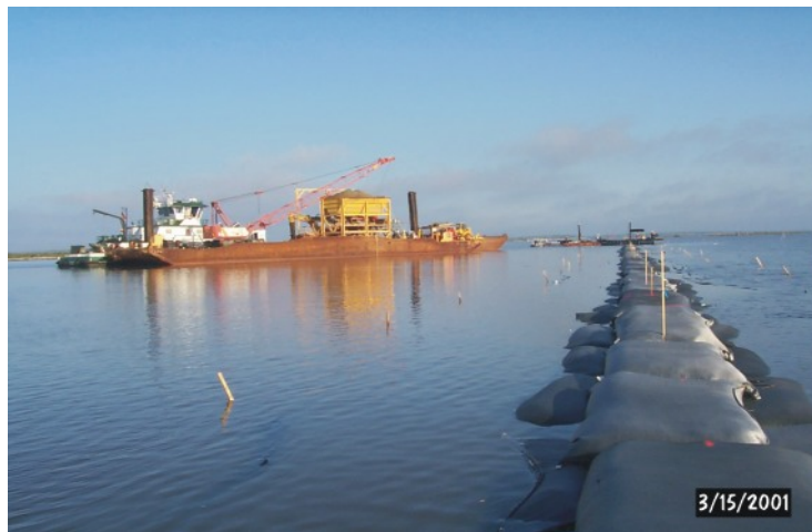
Geo-textile fabric bags were filled with a lightweight aggregate and then sewn closed. These bags act as the supporting core of the shoreline stabilization structure.
