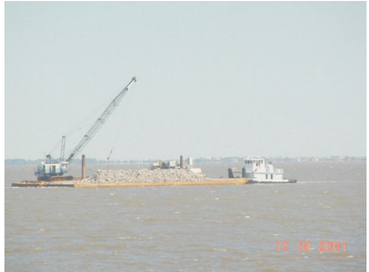
Fully-loaded barge of rock waiting to be unloaded at Bayou Chevee construction site.
